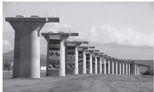
Note : The 1987.7 meters long Tsavo Super Bridge, with the highest point of 35.1 meters being constructed by China Road and Bridge Corporation (CRBC) will run over the Tsavo River and the existing meter gauge railway.
